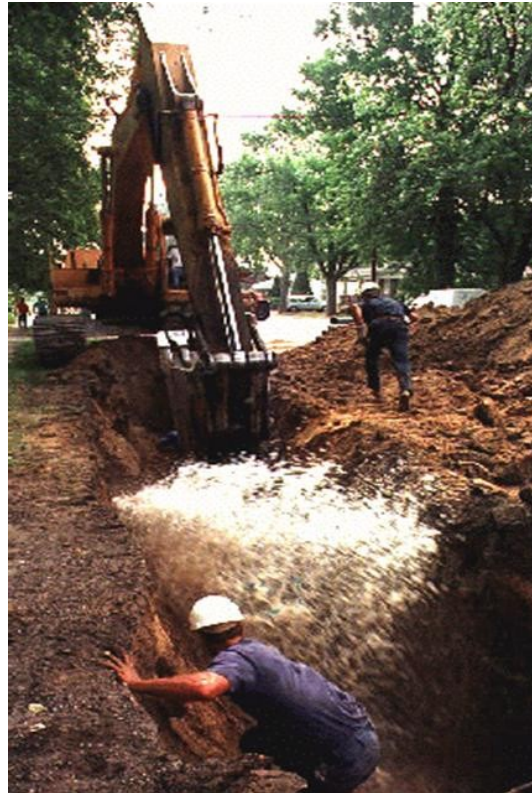
Workers escaping deep trench after a backhoe has burst a water main. While most trench fatalities are from cave-ins, drownings, electrocutions, asphyxiation and explosions are additional risks associated with water, sewer, gas and electric lines.
